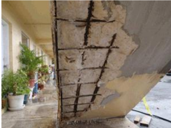
Cracked Stairs due to Freeze Thaw Cycles
